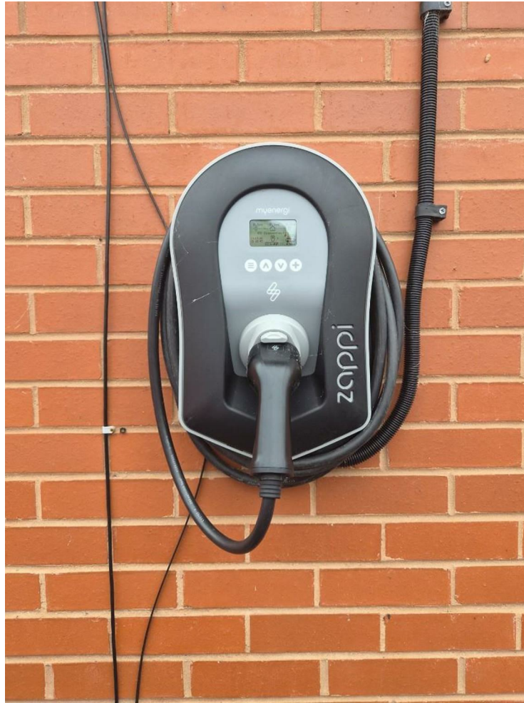
Car Recharging Point.
